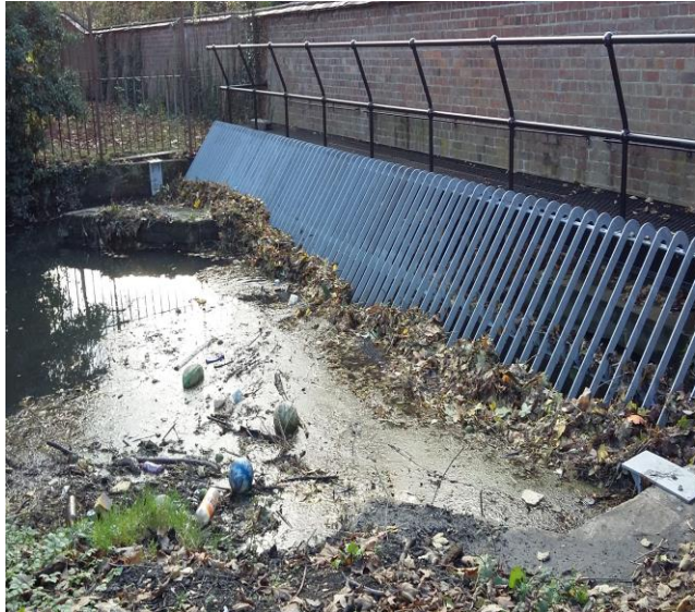
Figure 11: New trash screen after heavy rainfall
