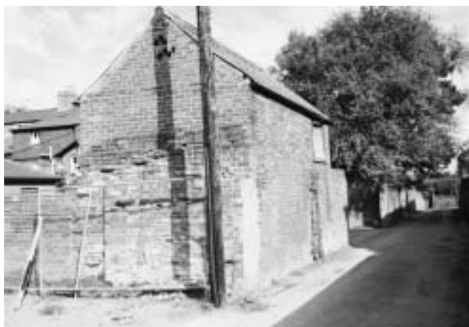
Development threatens the survival of the two 19th-century brick carriage sheds and stables to survive at the rear of properties in Royal Lane.
