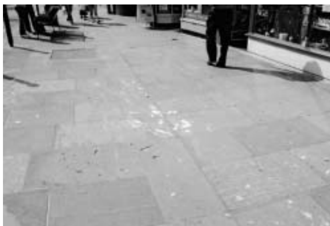
Paint spill damage to recently laid paving slabs on the corner of Northgate and Worcester streets.
