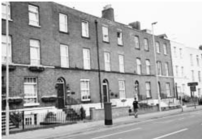
Unsympathetic alteration: replacement windows in Worcester Street.
