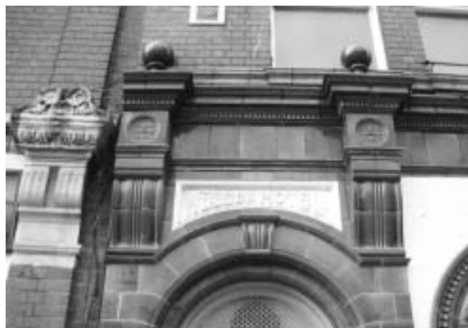
Detail of the glazed tiles at the former Wessex Hotel, Clarence Street frontage.
