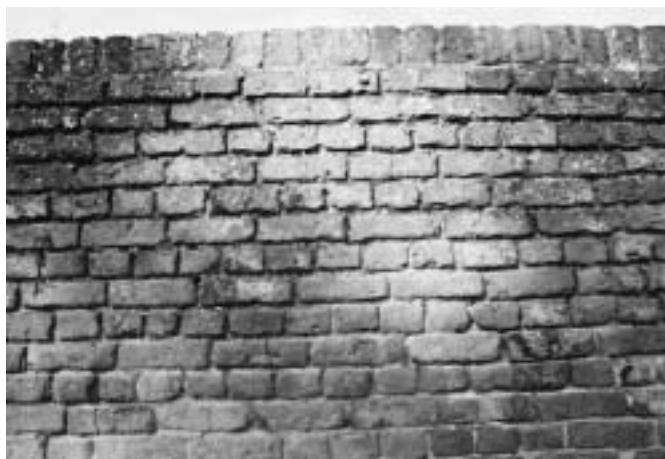
English bond brick walls along Hempsted Lane – possibly all that survives above ground of Hempsted Court, built c 1700.
